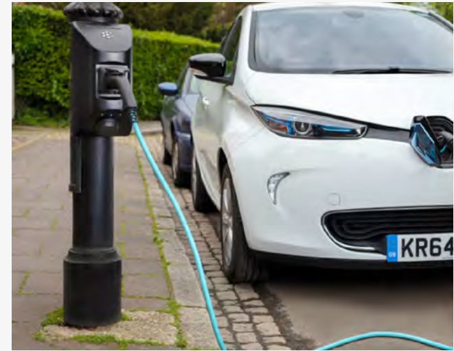
Figure 63: Example of on-street electric vehicle charging points.
